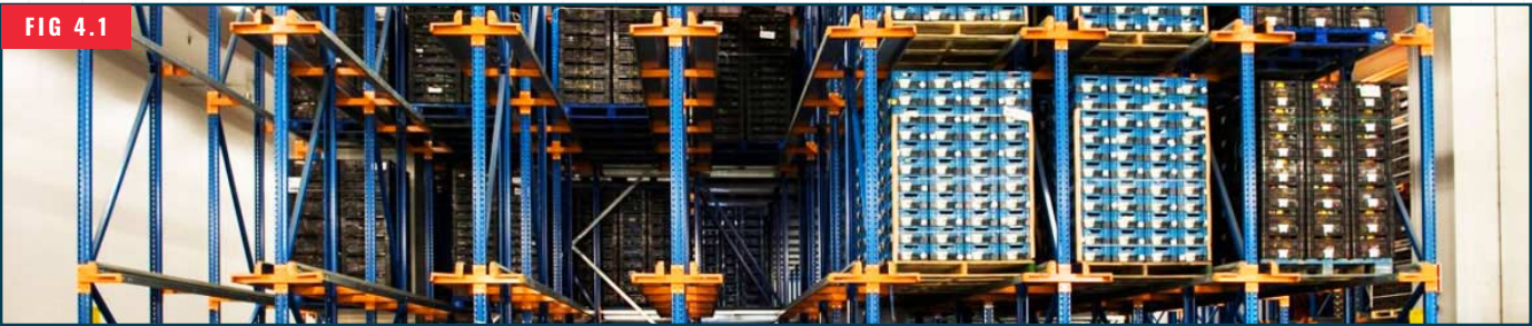
FIG 4.1 Hero shot of a completed, loaded install: clean aisles, straight rows, good lighting. The 'this is what you're buying' image, tied to the double-deep and 300,000 sq ft mixed new/used case studies that follow.
